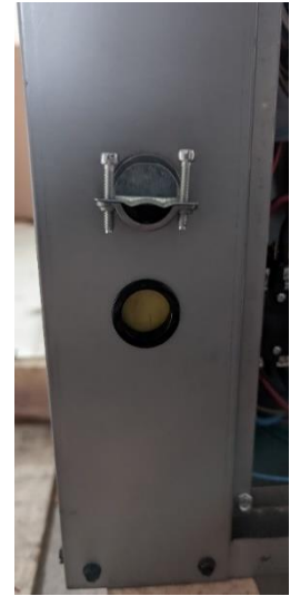
Figure 16: Main High Voltage wiring installation location on Heat Pump
