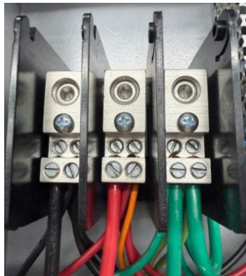
Figure 26: Electrical Main Outlets
